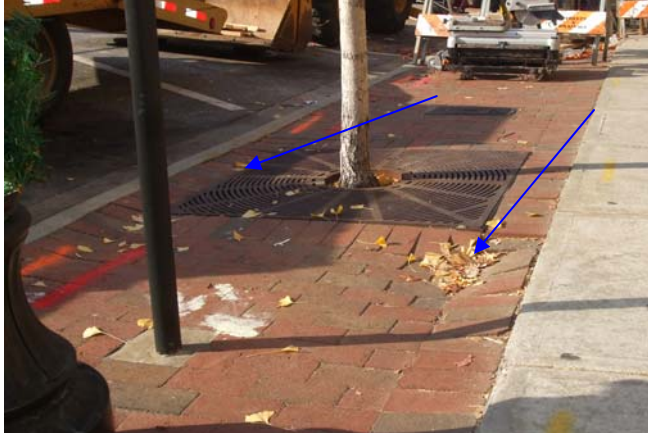
Figure 3. Collapsing pavers from improperly compacted structural soil.
